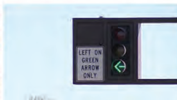
Protected Turn Lights
